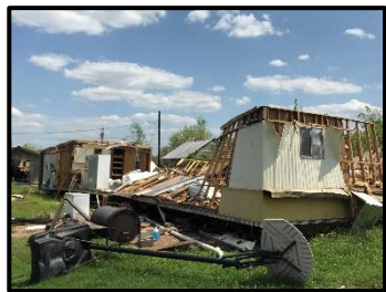
Above: Destroyed mobile home in Refugio County, TX during Hurricane Harvey in 2017.
